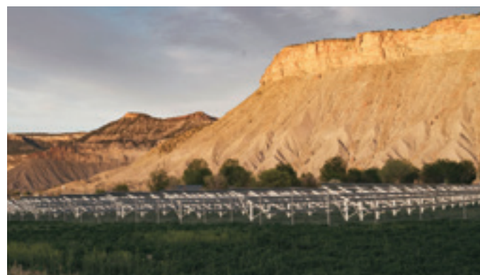
The Ute Mountain Ute Tribe invested more than $1 million in a new solar project and got a matching grant from the U.S. Department of Energy Office of Indian Energy. AVERY WHITE
