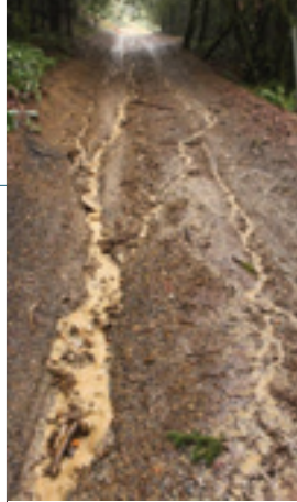
Water eroding an unpaved road delivers fine sediment to a creek in California. PACIFIC WATERSHED ASSOCIATES
