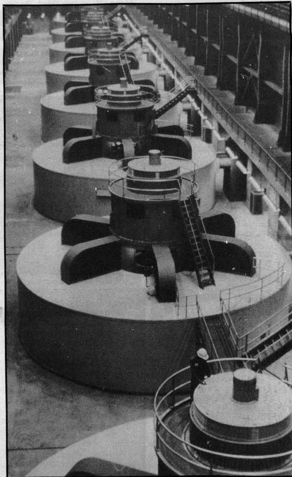
Glen Canyon power plant
