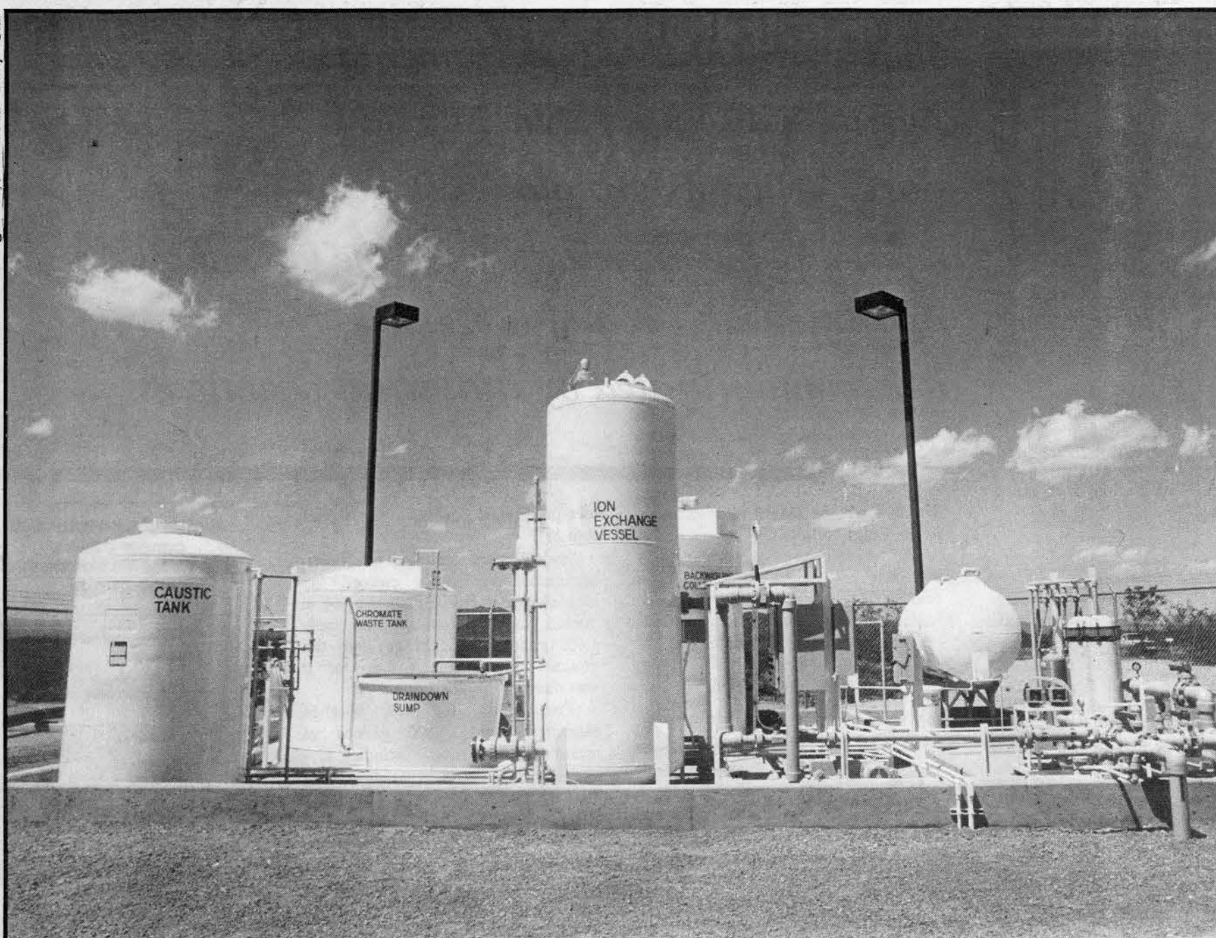
Small water treatment plant installed by Air Force at Hughes cleans chromium from groundwater
