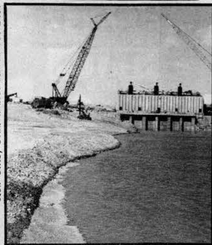
Hogup Ridge pumping station
