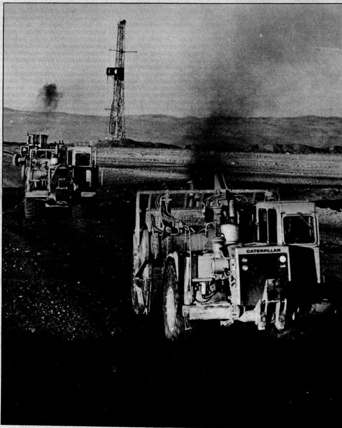
Sour gas facility in Whitney Canyon, north of Evanston, Wyoming
