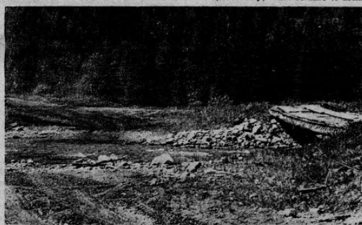
FORD AT CABIN CREEK. Trucks and bulldozers drive through the creek rather than upgrade the bridge to handle heavy equipment traffic.
