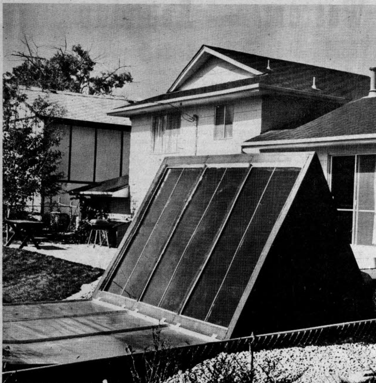
BACKYARD SOLAR FURNACE. A Nederland, Colo., firm has devised this style of solar furnace for homeowners with forced air heating systems. No need to dig a storage tank, the inventors say. The whole system is contained in this tidy unit. The firm, International Solarthermics Corp., says a small-size collector in a do-it-yourself kit would cost the consumer about $2,200.
