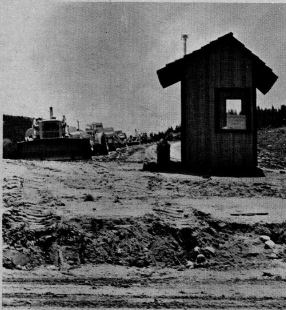
Mountains, valleys, and flowered meadows lie profaned before the onslaught of bull-dozers. Massive land developments and mountain subdivisions have hit the Mountain West without the adequate land controls needed to prevent environmental degradation.
